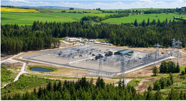
Blackhillock substation near Keith, Moray, which houses the HVDC converter station and synchronous condenser.
